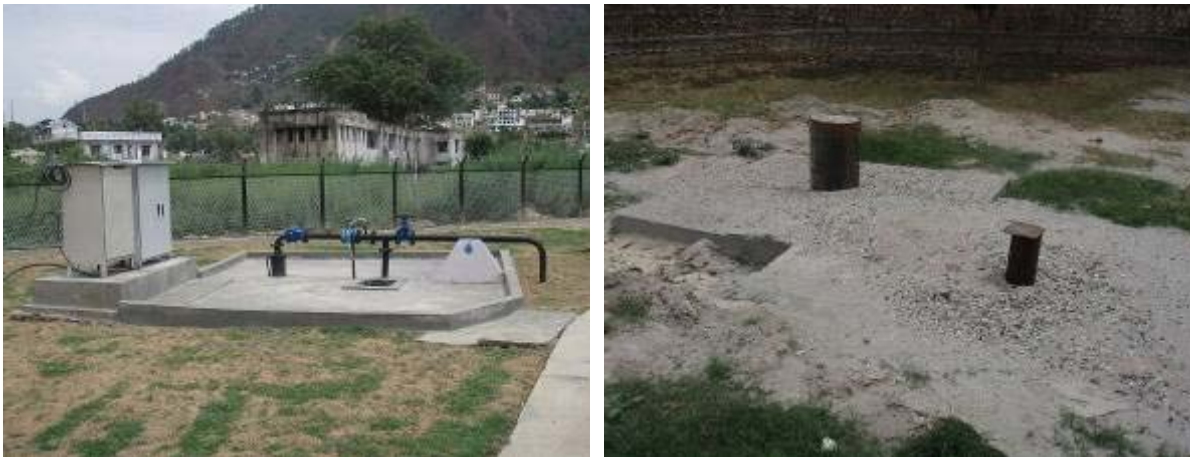
Figure 3-5 Sanitary sealing of production wells PW-DST (left) and PW5 and MW5 (right) at Srinagar RBF sites implemented by UJS (photos: Heinze and Lesch, 2012)
