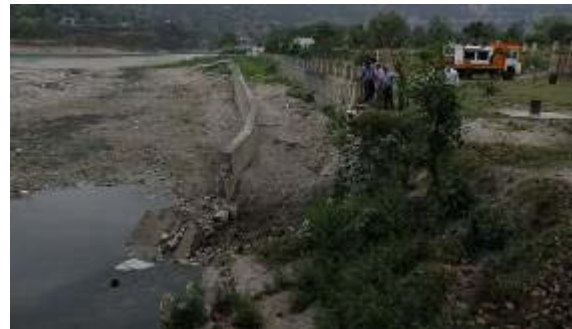
Figure 3-12 Damaged retaining wall of the RBF site in Srinagar after the monsoon flood of August 2011 (facing upstream) (Photo: T. J. Voltz, HTWD, 2012)
