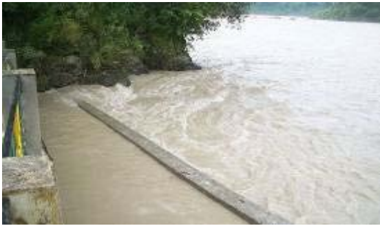
Figure 3-11 Intact retaining wall at the downstream-end of the RBF site in Srinagar at the onset of the monsoon flood in August 2011 (Photo: J. Ebermann, HTWD, 2011)
