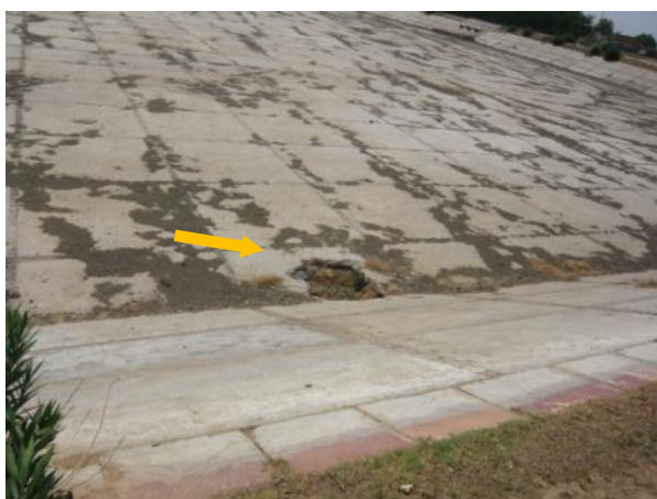
Figure 5: Hole in lining of FAP
