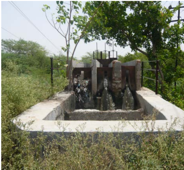
Figure 15: Partly blocked pre-treatment unit
