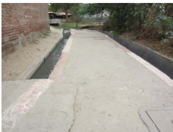
Figure 34: Pre-treatment unit below pavement
