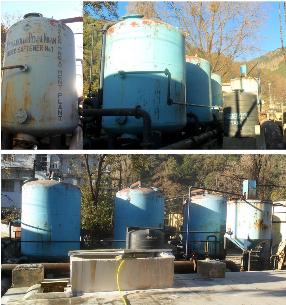
Figure 4 Ion-exchange water softening system treating bank filtrate at Nainital
