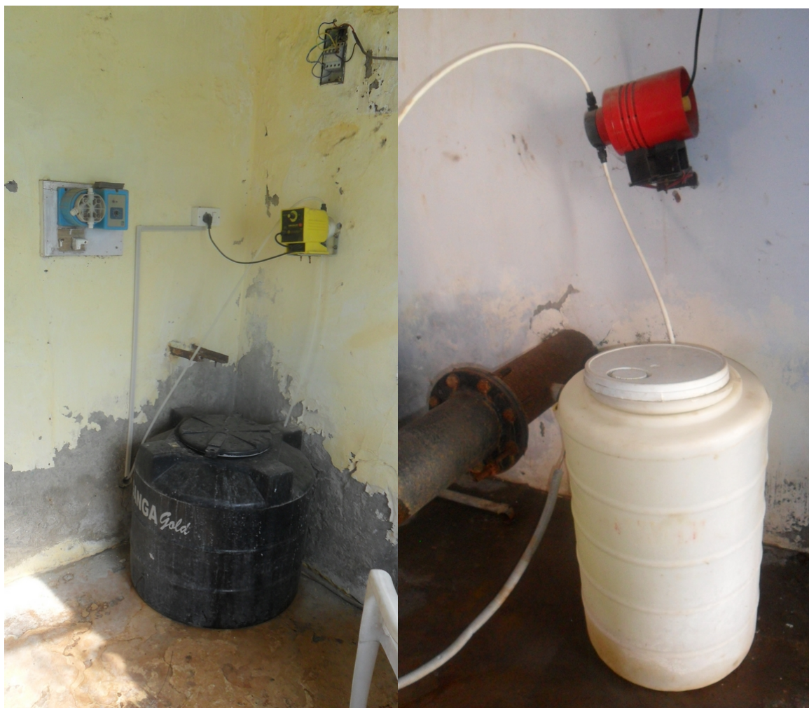
Figure 2 Typical sodium hypochlorite dosing system for RBF wells in Haridwar
