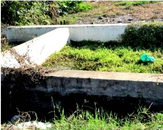
(C) Inadequately maintained pre-treatment unit at duckweed pond at Uncha, Roop Nagar, Punjab
