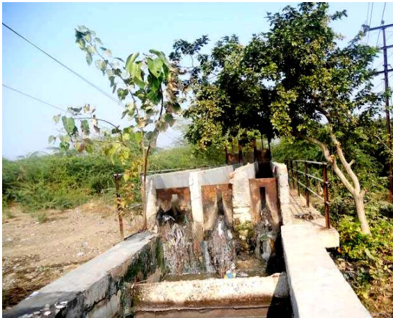
(C) Inadequately maintained pre-treatment unit at WSP based NTSSs, Mathura, Utter Pradesh
