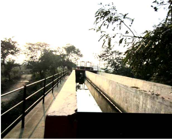
(A) Pre-treatment units installed at WSP based NTSSs, Agra, Utter Pradesh
