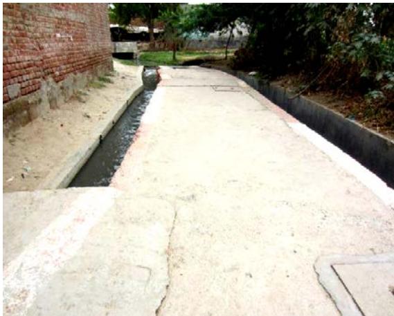
(A) Underground pre-treatment units installed at CW based NTSSs, Kachpura, Agra
