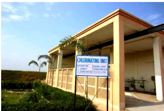
Picture 5: Chlorination unit installed for disinfection at UASB-PP, Agra, Uttar Pradesh, India
