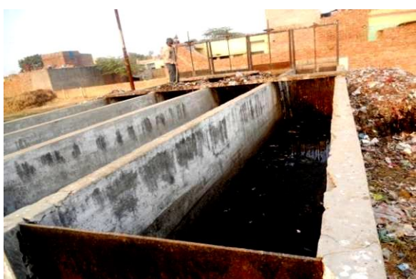
Picture 3.9 : Status of improper cleaning of primary treatment unit at site code; India_UP_6_WSP
