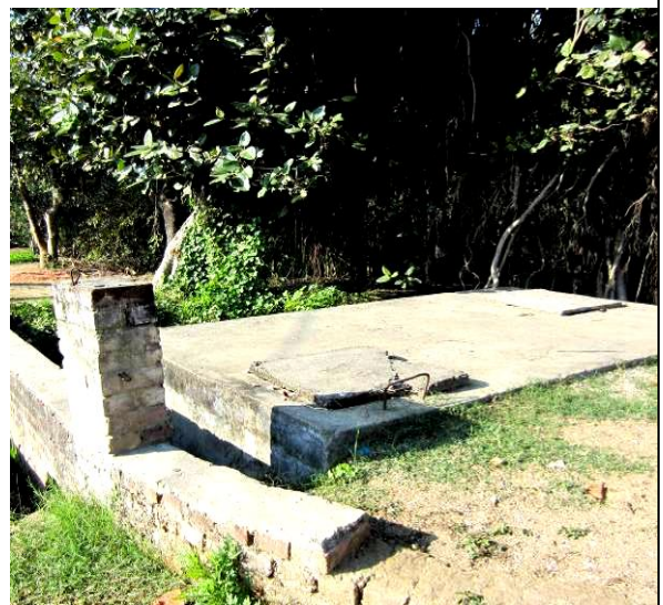
(A) Primary Treatment Unit
