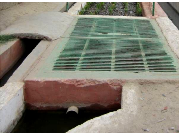
Picture 5.7: Treated wastewater collection tank cum pisciculture tank
