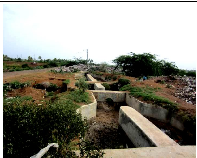
(A) Primary Treatment Unit
