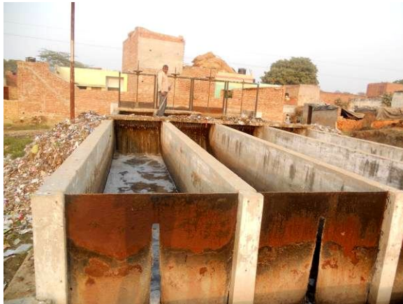
Picture 5.1: Manually removal of floating objects from bar-screen
