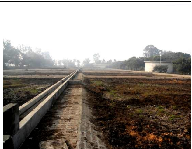
(E) Sludge Drying Beds
