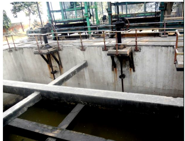
(A) Primary Treatment Unit
