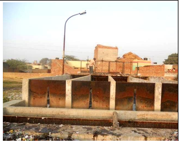
(A) Primary Treatment Unit
