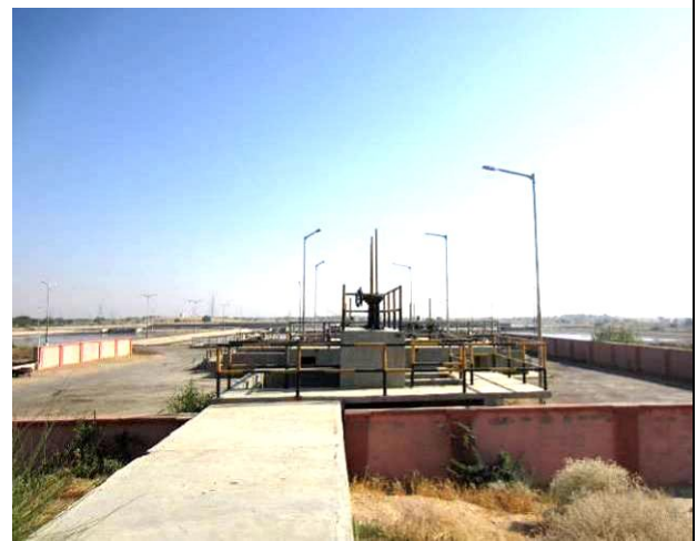
(A) Primary Treatment Unit
