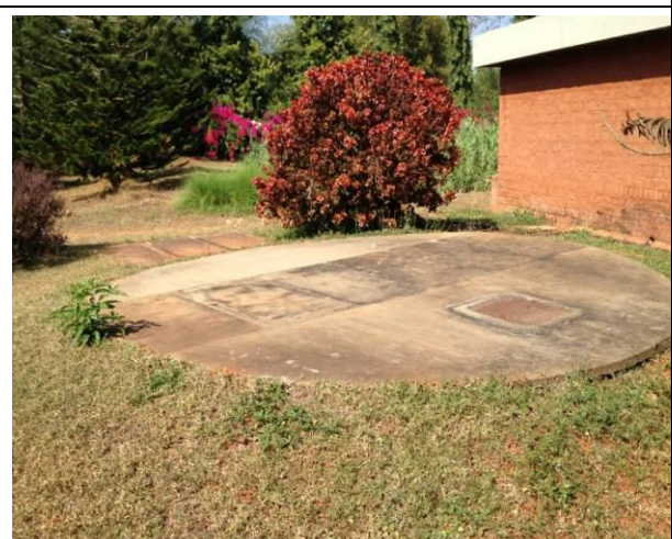
(C) Covered Imhoff tank
