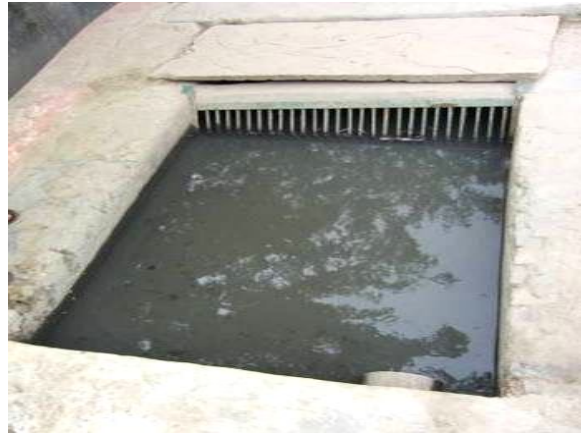
Picture 5.5: Open grit chamber for receiving wastewater from main channel
