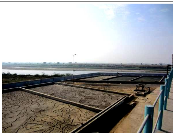
Picture 5.10: Mechanically sludge handling
