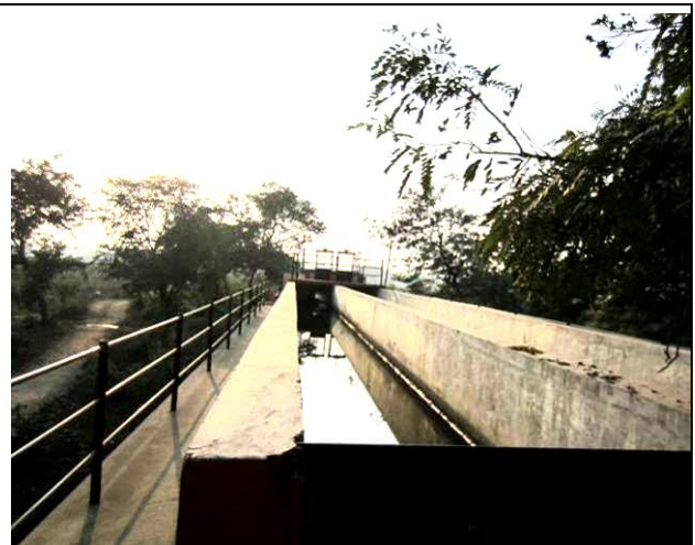
(A) Primary Treatment Unit
