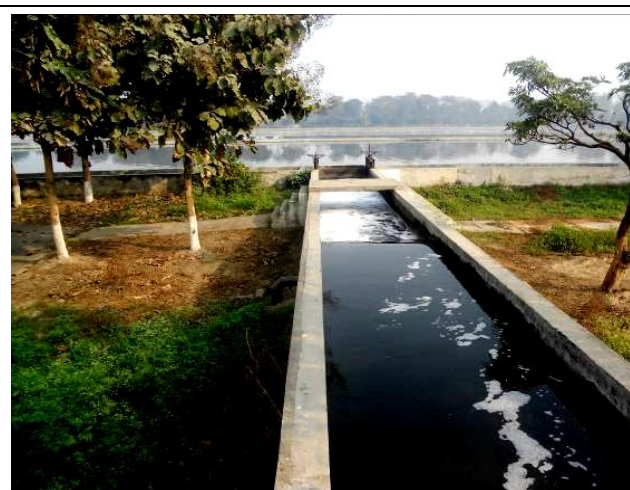
(B) Outlet of UASB
