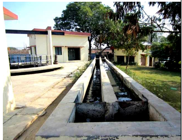
(A) Primary Treatment Unit
