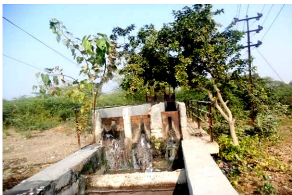
Picture 3.7 : Status of poor O&M of primary treatment unit at site code: India_UP_7_WSP
