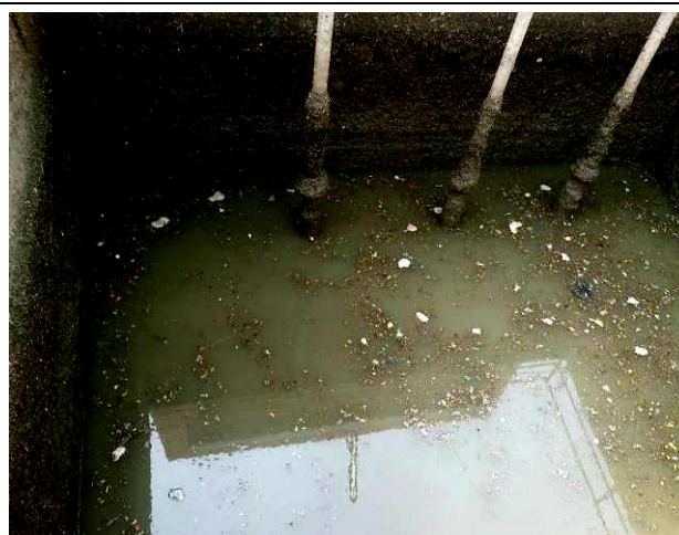
(A) Primary treatment Unit
