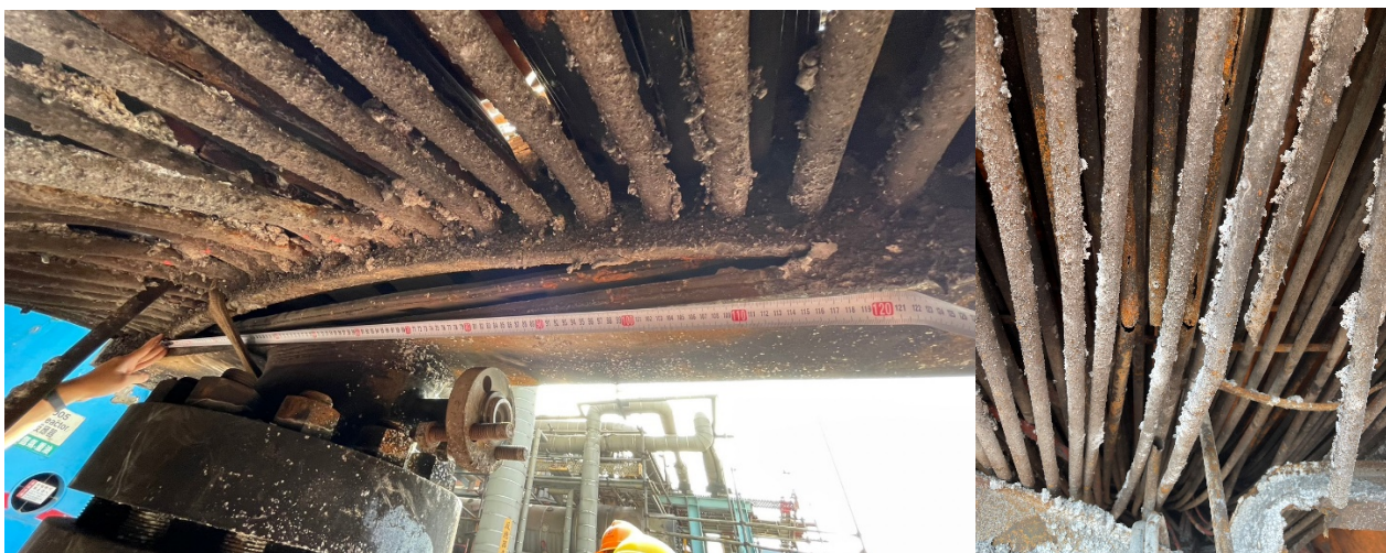
Fig. 4. Photo of the crack on E-3004A outlet header box and ruptured tubes
