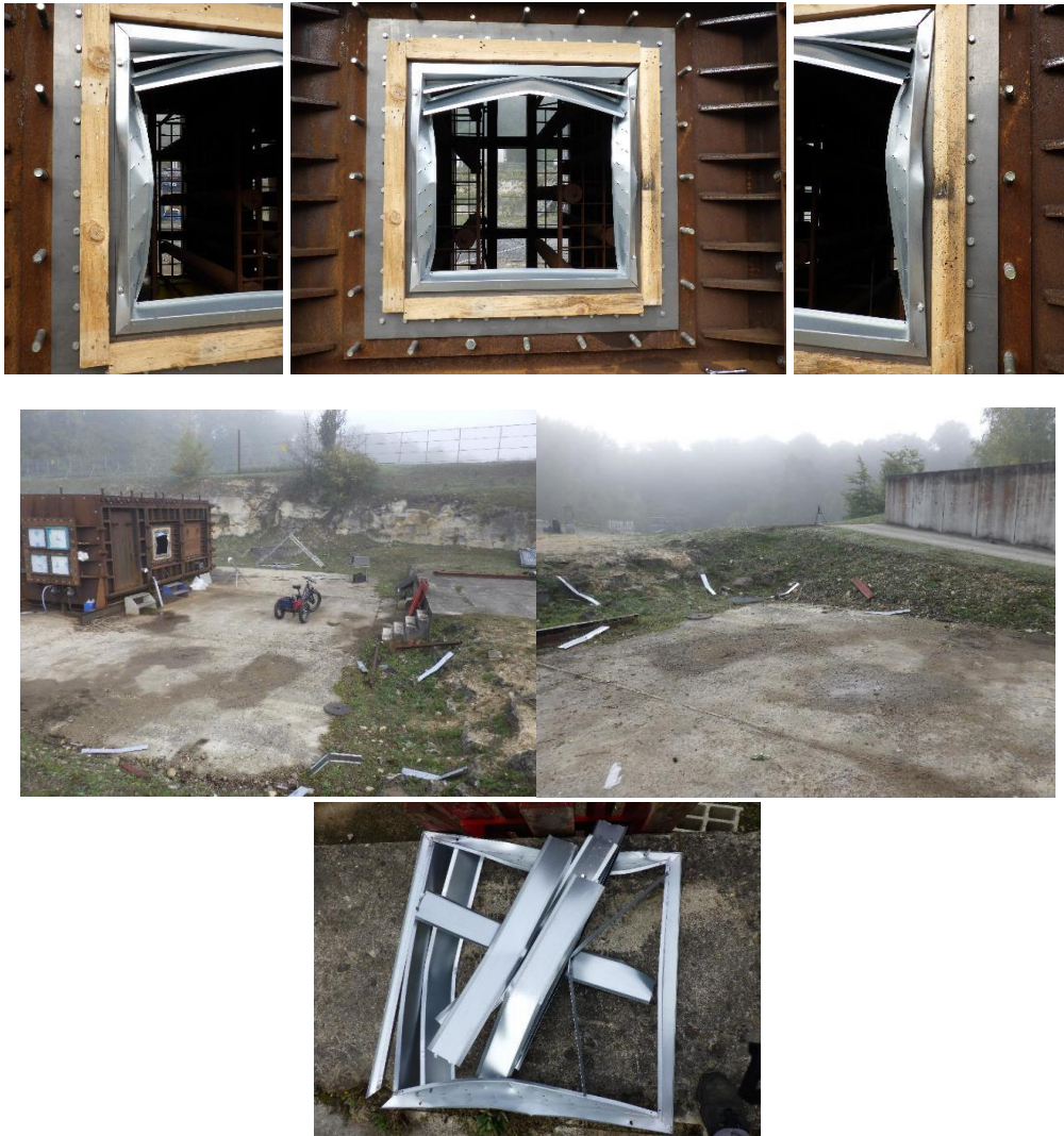
Fig 9. Images of the deformation of the grille frame holding the blades, the deformation and projection of the blades - Grille 0.8 \times 0.8 \text{ m}^2 at 100 mbar
