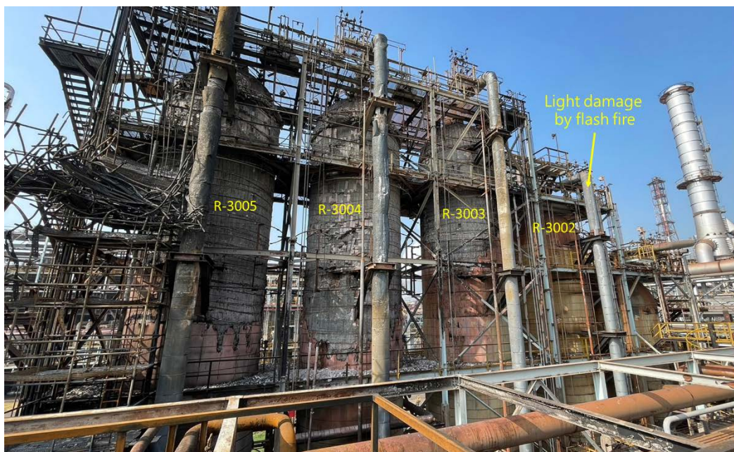
Fig. 1. Photo of damage on RDS reactors
