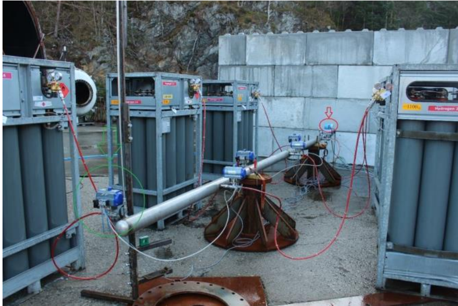
Fig. 1. Overview photograph of the gas supply manifold system, showing the gas supply skids, their high-pressure hoses (red hoses), the pneumatically actuated ball valves (circled in green) and Coriolis flow meter (circled in red).
