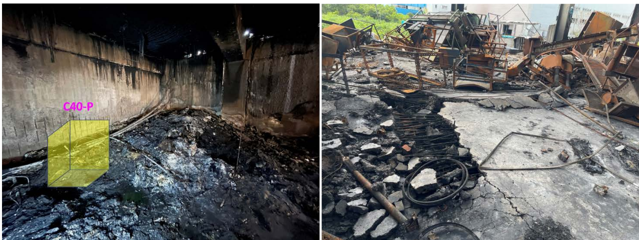
Fig. 8. Damage of warehouse interior (left) and ruptured floor on second floor (right)
