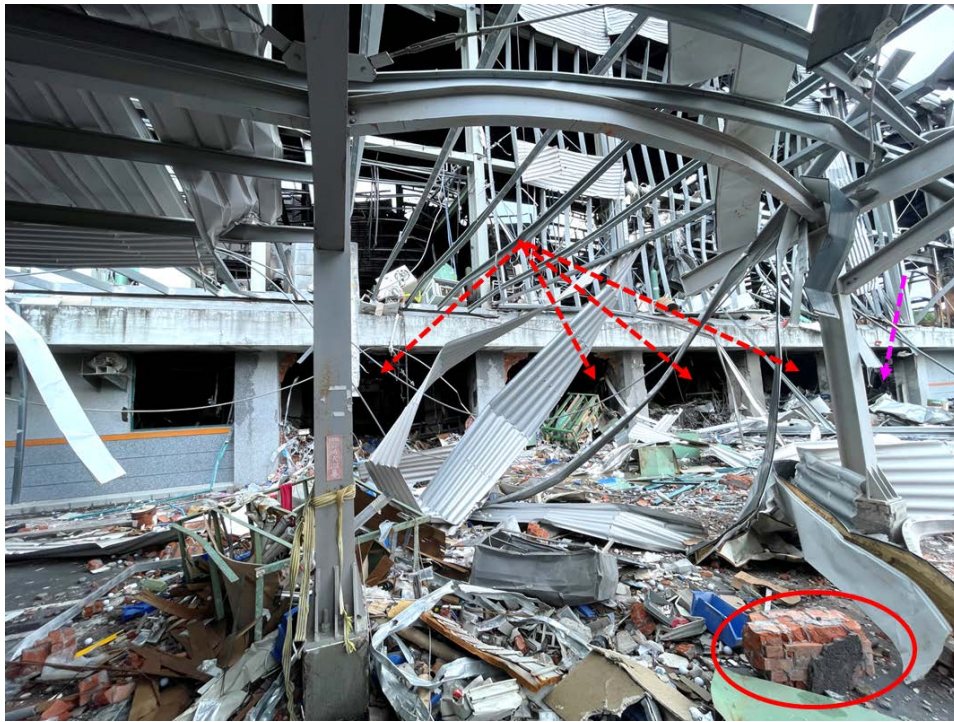
Fig. 7. Damage of the plant exterior. The 4 red arrows indicate the brick walls that were blown away. The red circle is a fragment of brick wall. Pink arrow indicates the entrance of warehouse
