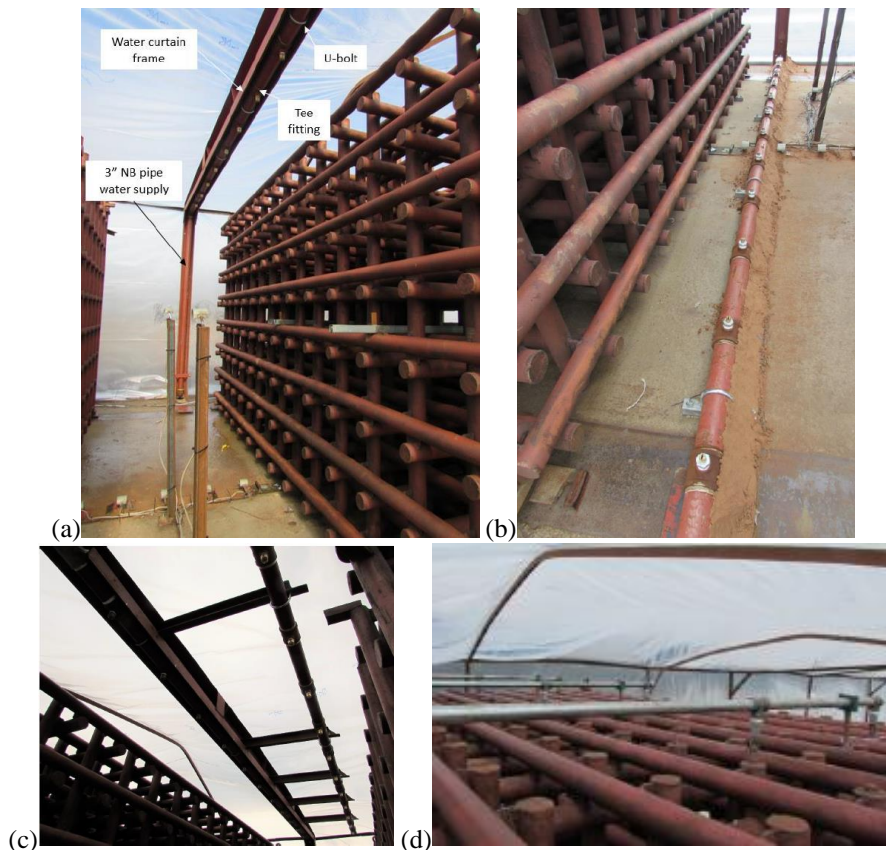
Figure 6: Example of water curtain arrangements. (a) Single curtain (in middle of gap), (b) upwards curtain, (c) double curtain, (d) general area deluge
