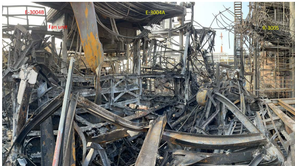
Fig. 2. Photo of damage on E-3004A/B REAC and nearby steel structure and pipeline
