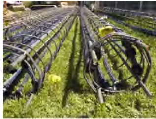
30m Energy Piles
