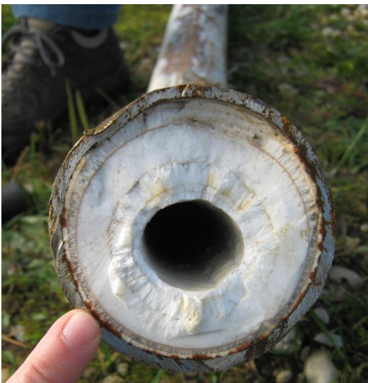
Figure 20 Carbonate scaling in Benedikt as occurred during testing of the well
