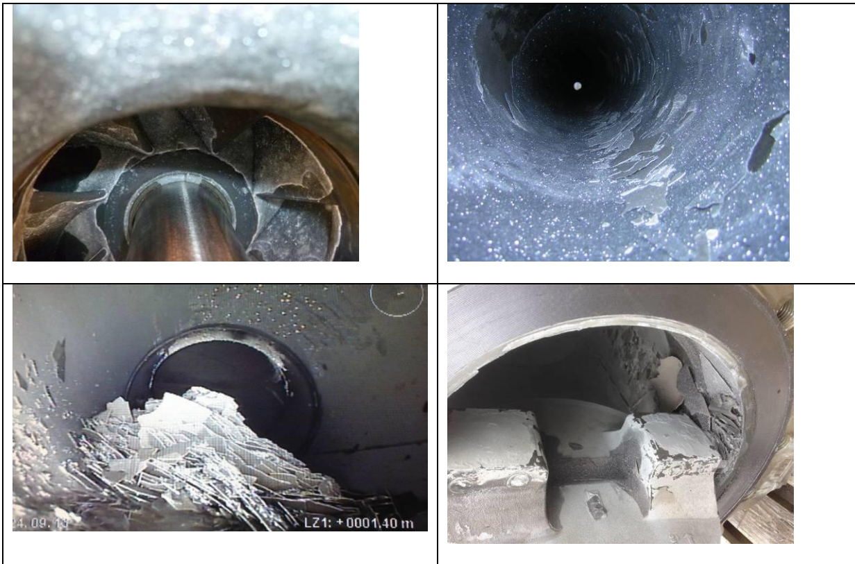
Figure 23 Carbonate scalings in (a) a pumping stage of the ESP (b) rising pipe, (c) surface pipe and (d) heat exchanger of four geothermal power plants located in the Bavarian Molasse Basin.
