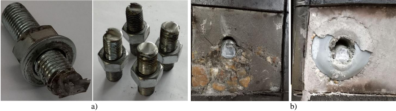
Fig. 5 a) Ductile failure of the bolts and b) failure of the concrete (left) and the mortar filling (right) with the bolt deformation
