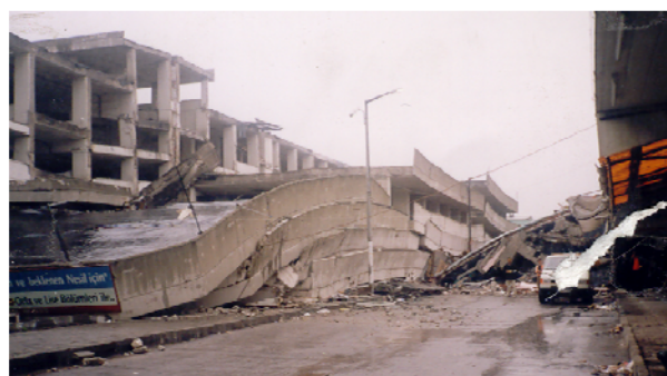
Fig. 1 A seriously damaged RC building in Marmara region
