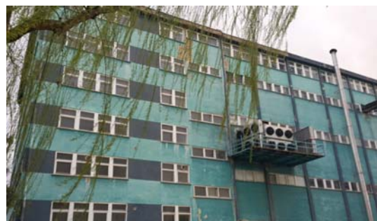
Fig. 9 Weak framed typical official building in Turkey
