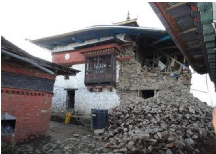
Figure 2: Damaged temple after earthquake (September 18, 2011) in Bhutan. Photo courtesy of British Library Endangered Archives Programme.
