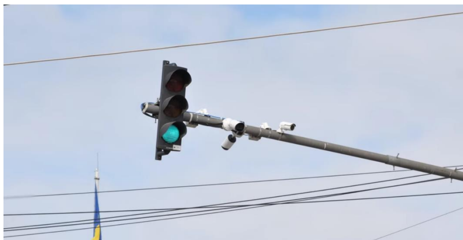
Figure 21. UC4 Cameras installations.
