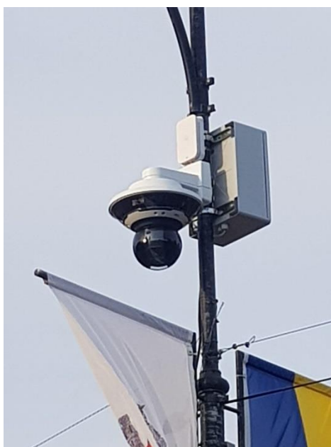
Figure 19. UC1 Cameras and 5G CPE installations.
