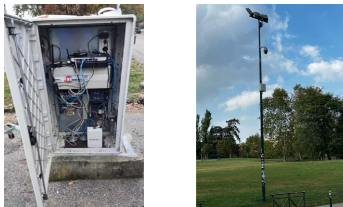
Figure 6. Installed sensors (left) and pole sensors (right).
