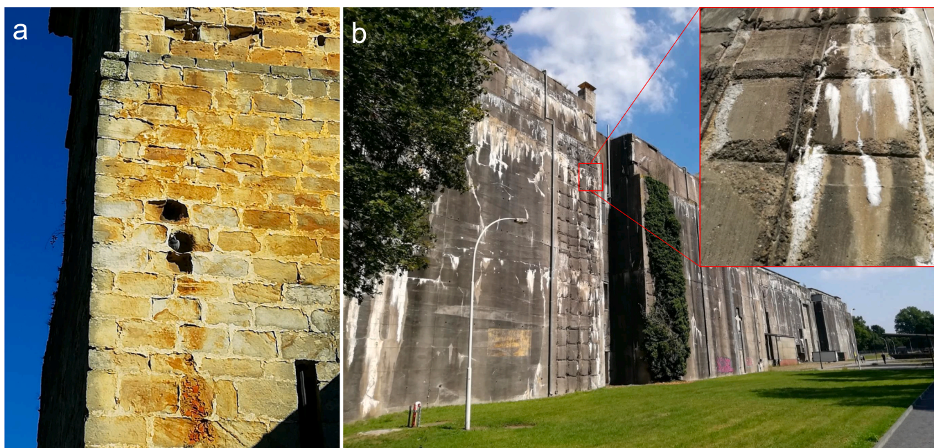
Fig. 1. Lime carbonation: positive and negative effects. a) Masonry structure of the XIIth century Colegiata of Santillana del Mar (Spain) built using sandstone blocks and aerial lime mortar; b) the deleterious effect of delayed carbonation of a reinforced concrete structure (II World War submarine bunker Valentine, Bremen, Germany). Massive loss of concrete scales associated with steel bar corrosion upon carbonation is observed, along with carbonate efflorescence/encrustation (white stains). See detail in inset.
