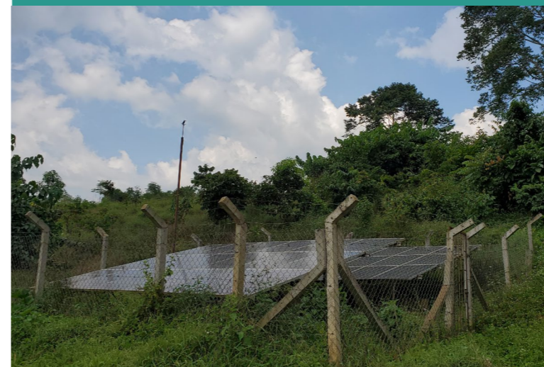
Figure 12. Solar powered system installed at Nkokonjeru Area Cooperative with support from Ugandan Government
