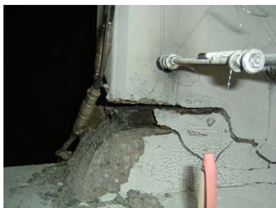
Fig. 3 Fallen state of the parts of the concrete at the upper corner of the corbel of the DP1R specimen
