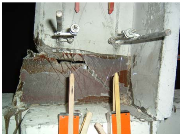
Fig. 2 A view of corbel and bottom side of the beam at the CP1R specimen after experiment
