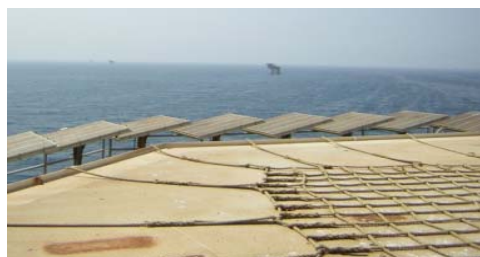
Fig. 2 Solar panel on unmanned platform
