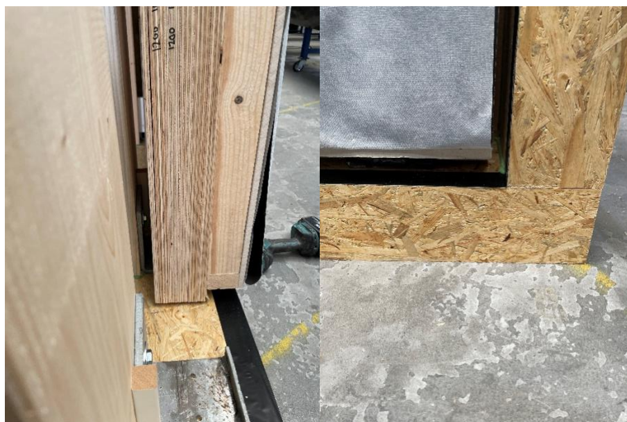
Figure 10: Placing the two lower elements: on the left the e-PANEL, on the right the e-CLT panel
