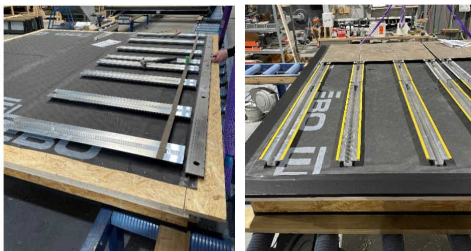
Figure 15: Placing the facade supports, waterproofing the front of the test cabinet and placing tiles
