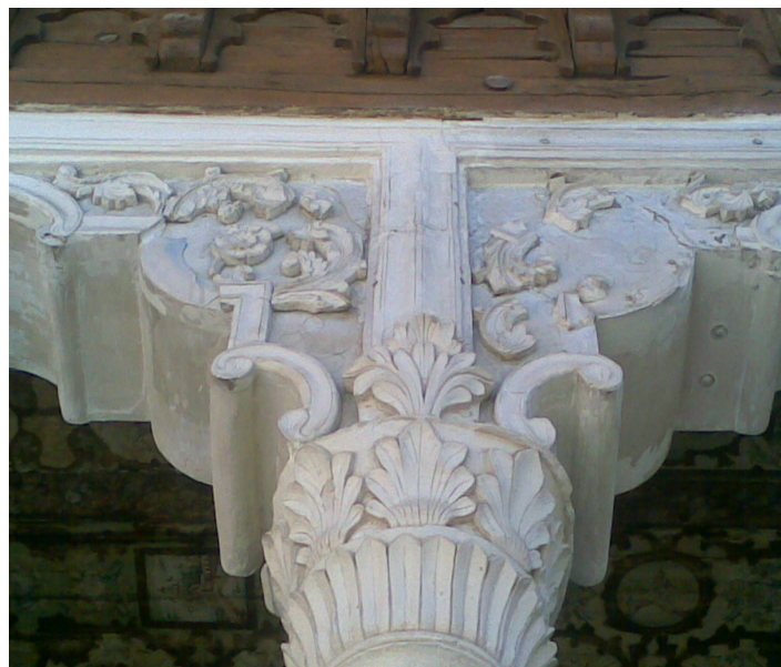
Fig. 3 Damage to the historic building of temperature and humidity changes
