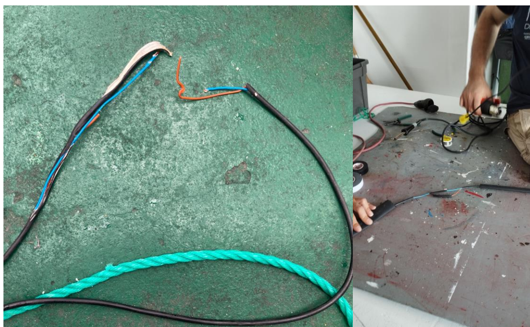
Figure 22. The aspect of the electrical cable after getting trapped in the plates of the winch, and the team working to repair it whilst the Azor drift-cam was being deployed using the spare umbilical
