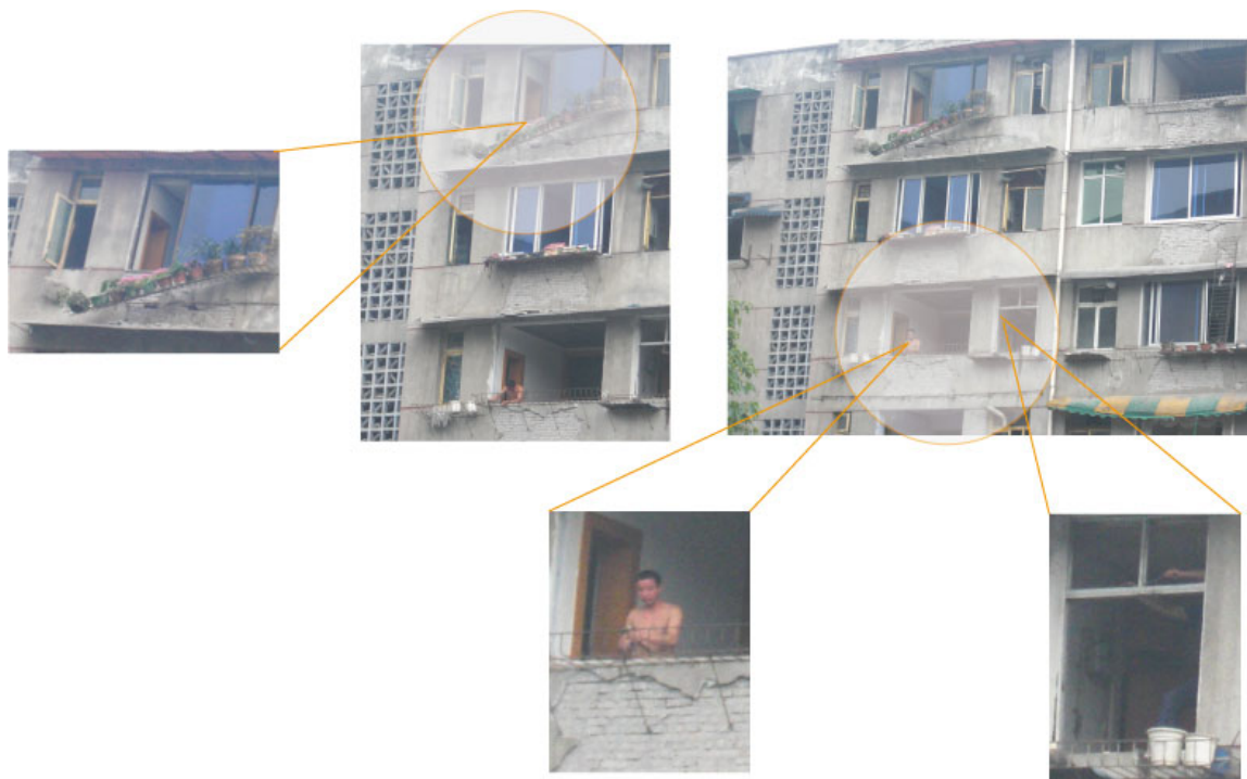
Photograph5. Danger posted by the Falling Objects
