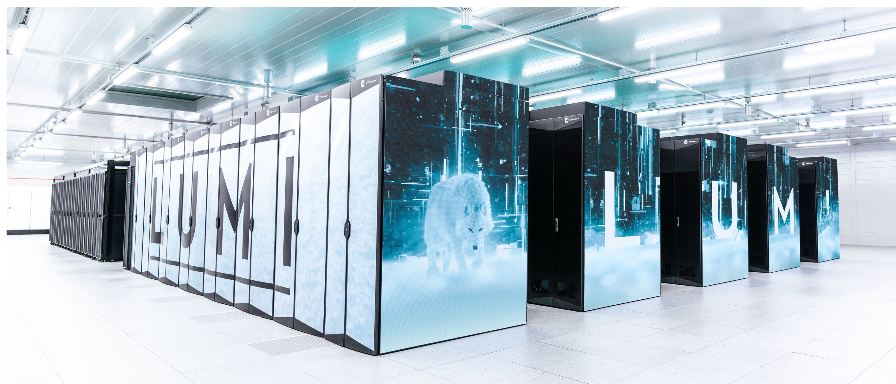
Figure 1. Cabinets of the LUMI supercomputer.
