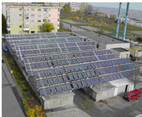
Fig. 4 Solar thermal system in Mangalia city
