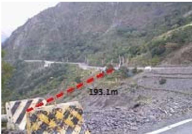
Fig. 1 Location of slope collapse and sliding
