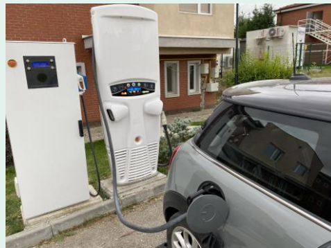
Figure 89: V2G and DC Chargers
