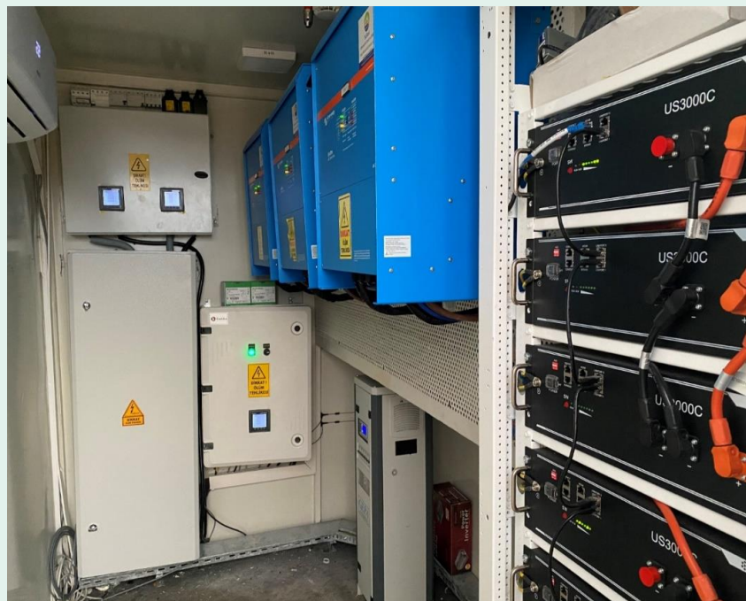
Figure 90: Energy Storage System 2: 45kW 32kWh
