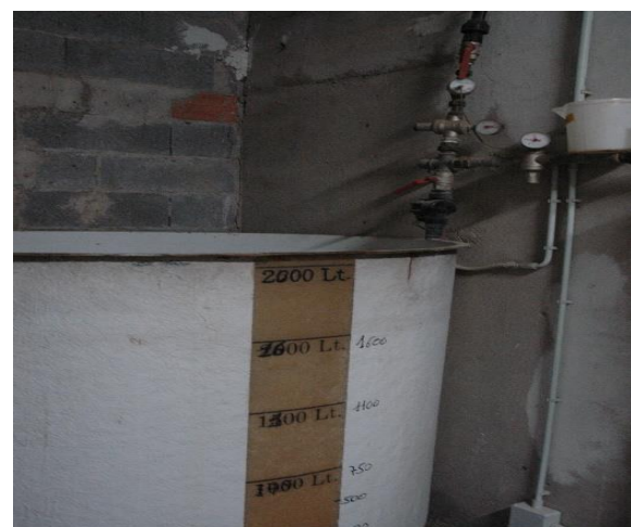
Figure 5. Example of emergency water system (IZSLER)
