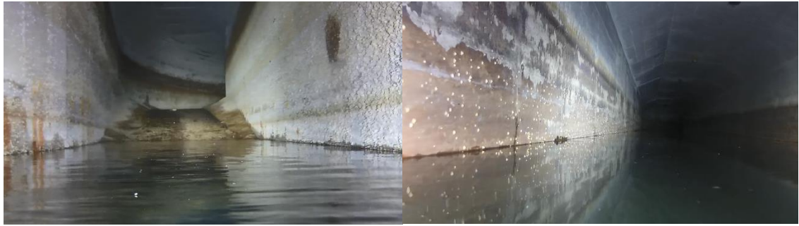
Figure 3 - Example of a visual inspection of a tunnel in a power plant
