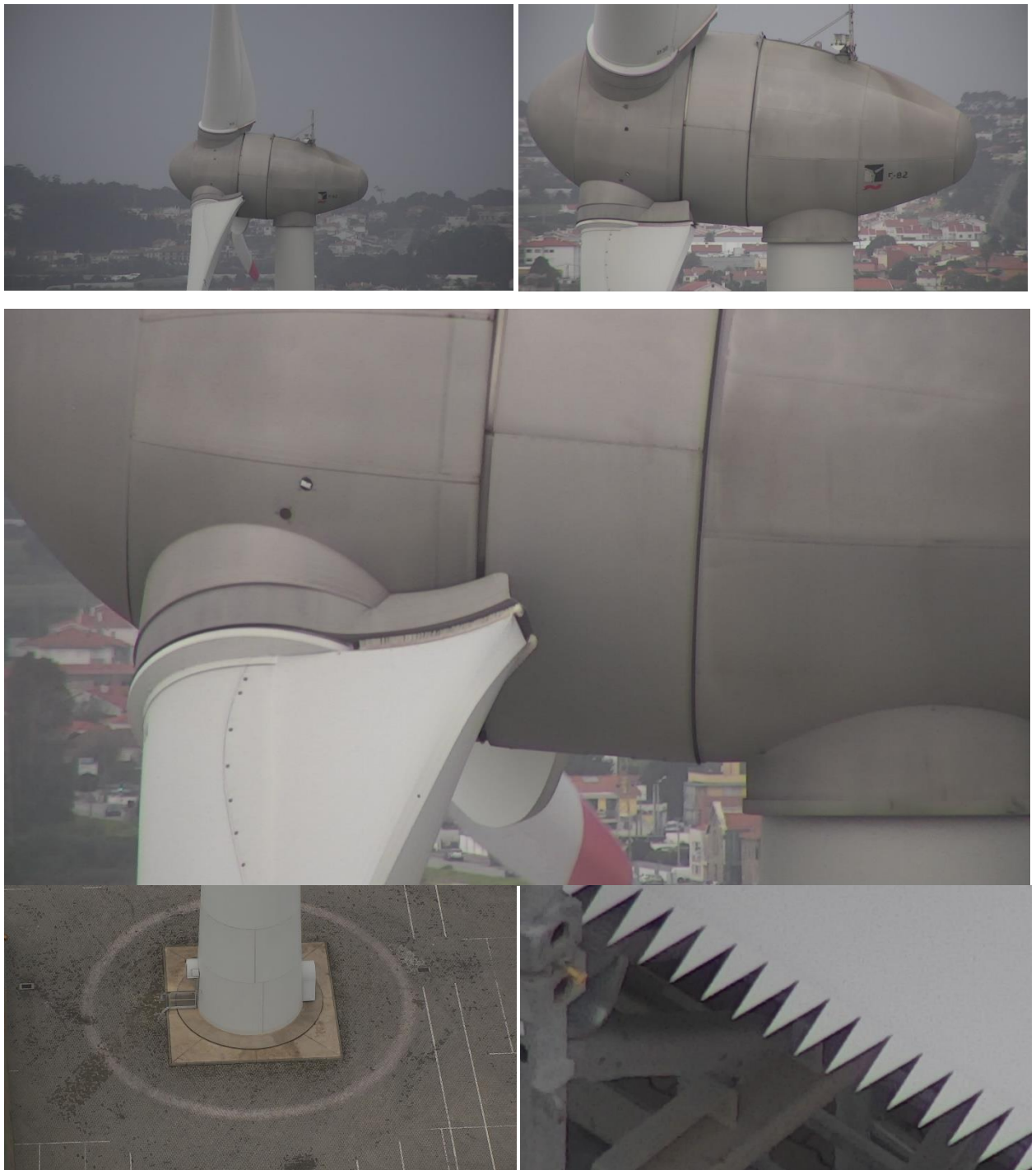
Figure 6 - Images taken from a visual inspection of the blades of an offshore wind turbine
