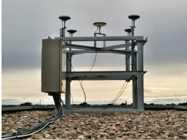
Fig. 2. GNSS antennas at the roof of CTTC's headquarters.
