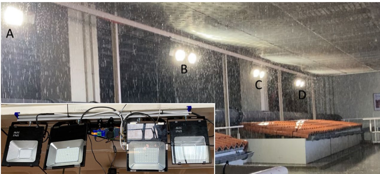
Figure 1. Installation of cameras based on Raspberry Pi and lamps in BLOCK. Four positions distributed along the facility were selected to hold two different image acquisition systems and LED and UV lamps.
