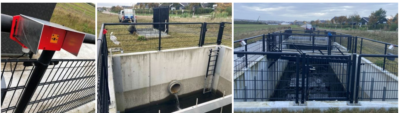
Figure 1: Installation of the equipment at the Experimental SUDS facility.
