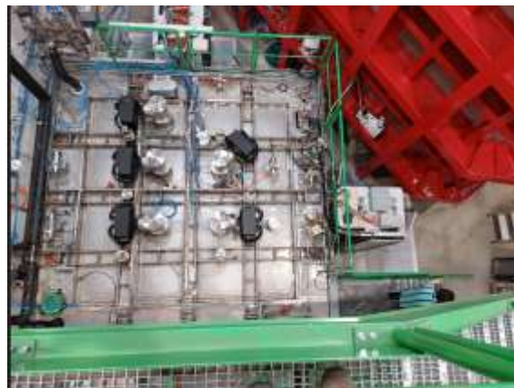
Fig. 6: Cold-Box roof top view during CRP2 operation with 5 chimneys each one cabled to a uTCA digitization crate (black boxes)
