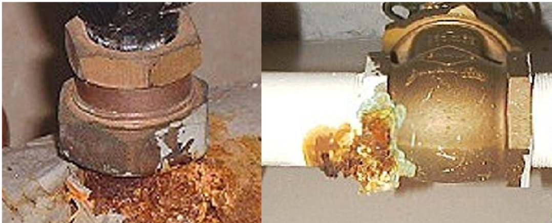
Fig. 5-21. Galvanic corrosion in steel connected to copper.
