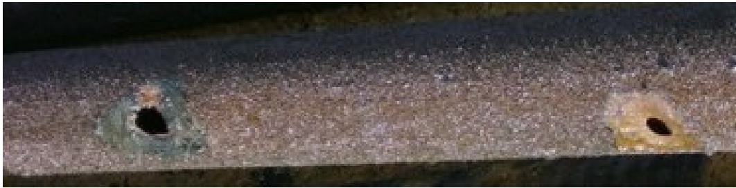
Figure 5-6 Pitting corrosion in water well tubing.
