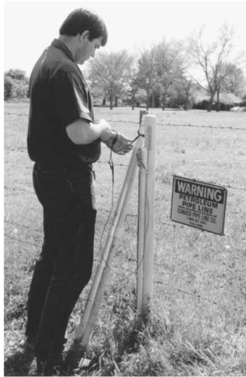
Figure 9.20 Test station with an electrical connection to the pipeline.
