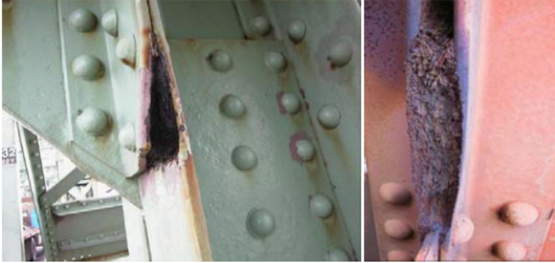
Fig. 5-18. Pack rust corrosion
