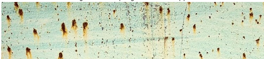
Fig.5-8B. Pitting corrosion in stainless steel sheet.
