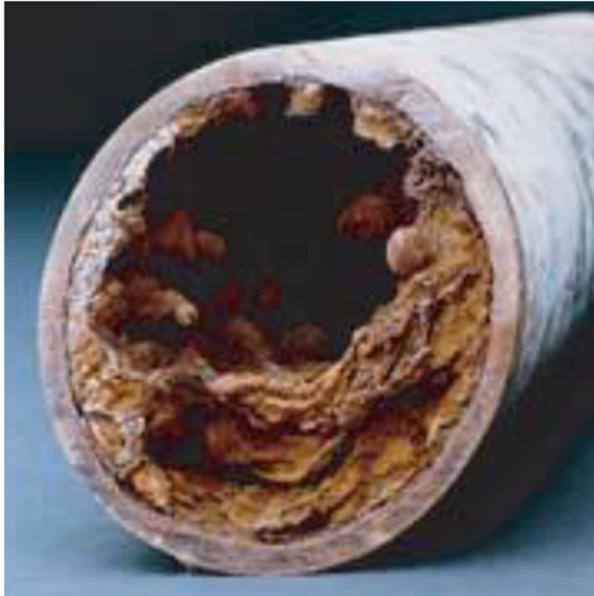
Figure 11 Pipeline affected by MIC corrosion.
