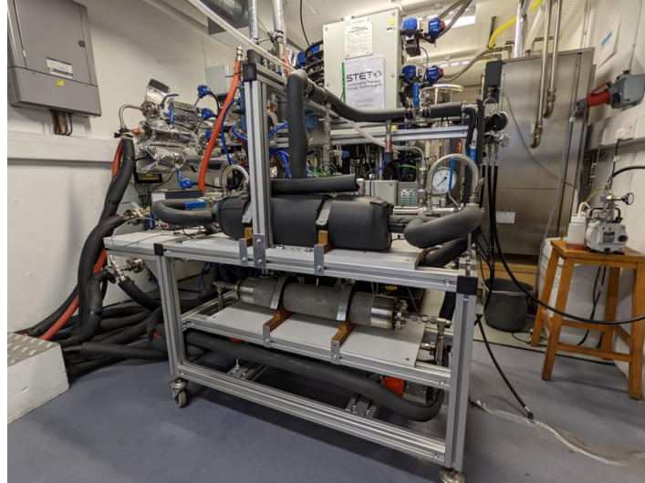
Figure 4. The completed resorption test bench situated in front of the ThermExS testing facility. The LTS reactor (NaBr) is situated on the top shelf (insulated), with the HTS reactor (MnCl 2 ) on the middle shelf (stainless steel shell visible, uninsulated).
