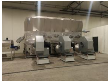
Fig. 9. Industrial scale pulsed fluidised bed dryer.
