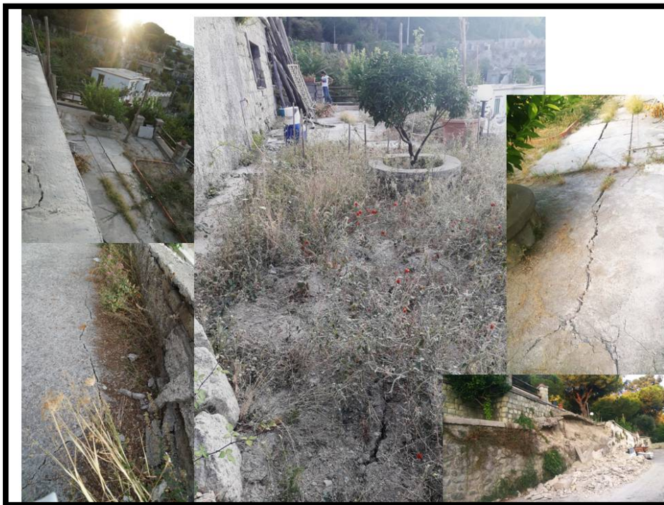
Picture 2: System of parallel surface coseismic fractures and drywall sliding in via Montecito (Casamicciola).
