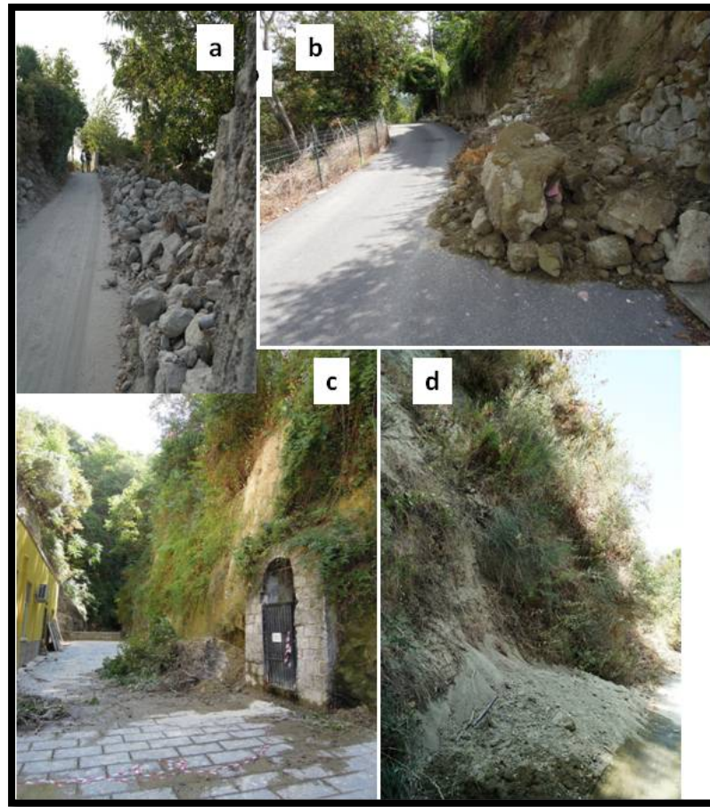
Picture 3: Collapse phenomena of drywalls at Casamicciola, in via dei Carri, (a), and in via Nizzola (b); Small landslides in volcanoclastic deposits in via Nizzola (c) and in via S. Barbara (d).
