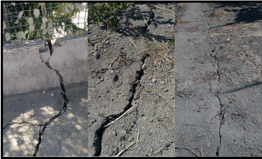
Picture1: Coseismic fractures in via Crateca, Fango locality (Lacco Ameno).
