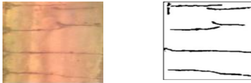
Figure 3: Original and Processed Images: Linear Cracks.
