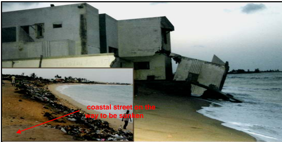
Photo 2: Certain damages caused by coastline erosion in Benin (March 2005)
