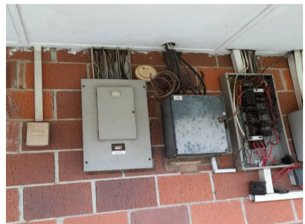
Plate 3: Fire alarm located at the electric distribution board. Source (researcher’s fieldwork, 2022)
