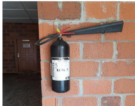
Plate 2: Portable fire extinguisher. Source (Researcher’s Fieldwork, 2022)
