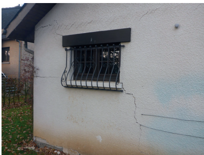
Figure 6: Cracks typical of a shrinkage-swelling phenomenon.
