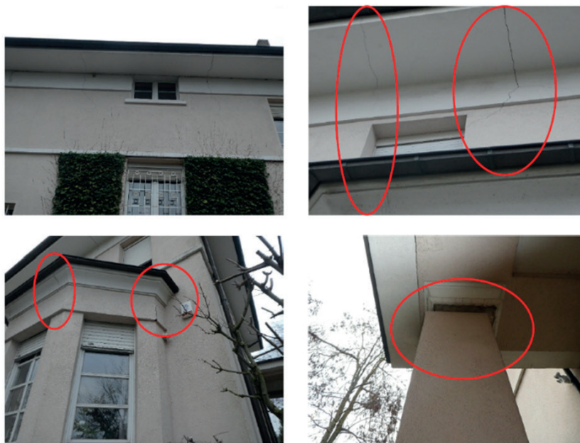
Figure 10: Cracks in the walls and rotation of the entrance pillar.
