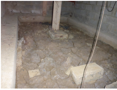
Figure 5: Desiccation crack inside a ventilated void of a house without a basement. The clays are totally dry on the inside, but their water content continues to vary on the outside, causing differential settlement and the appearance of cracks.
