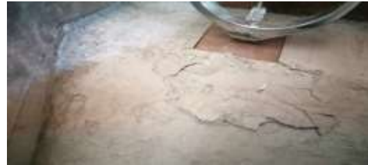
Fig.5:-Failure of slope
