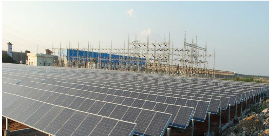
Fig. 3. Installed and fully operational 1 MWp utility-scale solar PV plant at Revulapally (Village), Mahabubnagar (District), Telangana (State), India (Kumar et al., 2018).
