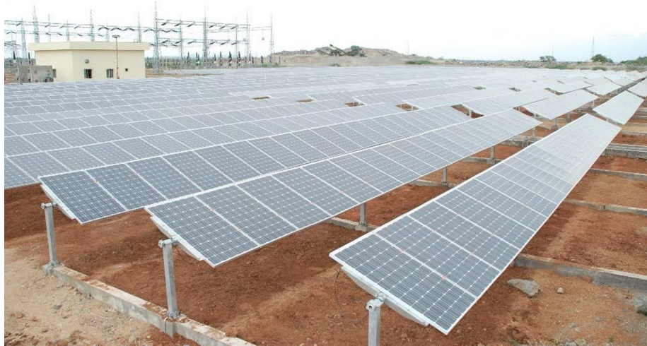
Fig. 1. PV modules on to the mounting structures in strings each consisting of 21 PV modules.
