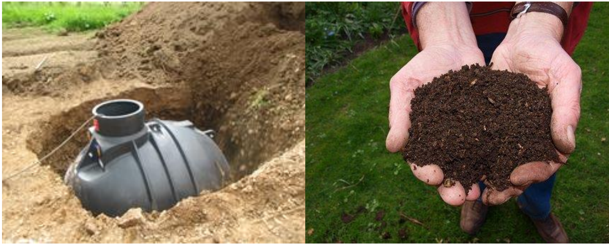
Figure 12: Sludge storage tank (left) (photo: U.Strniša) and compost (right) (photo: pixabay)
