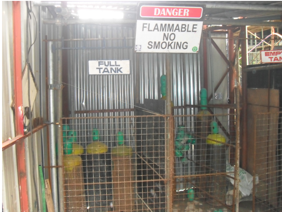
Figure 16: Proper Storage of Fuel tank
