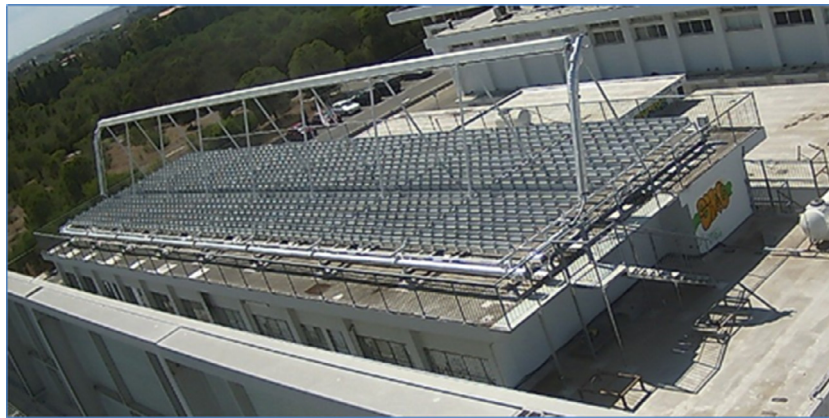
Fig. 12. The Linear Fresnel system installed on the roof of adjacent school.
