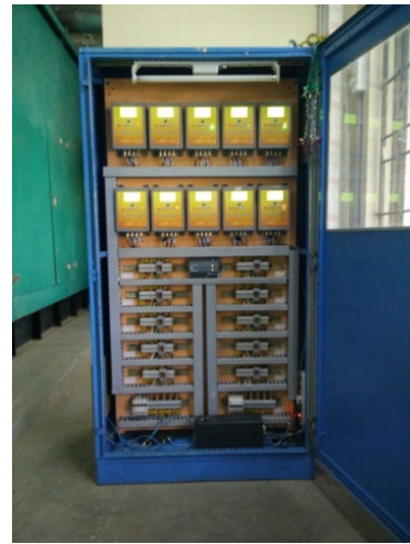
Fig. 14 View of the developed system installed in the field
