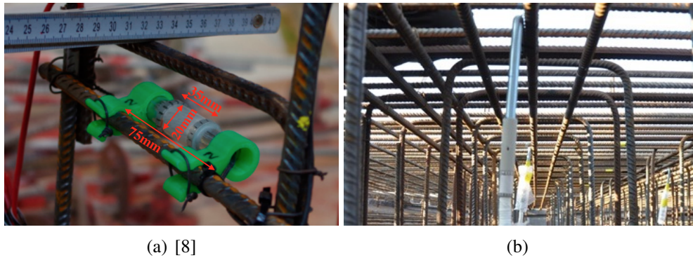
Figure 3. (a) Mounting SO807 to reinforcement with 3D-printed adapters on new bridges; (b) Mounting SO807 with L-shaped rebar on Gliwice bridge.
