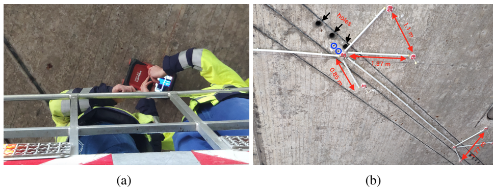
Figure 6. (a) Detecting rebar by GPR (Ground-penetrating radar); (b) Real position of the sensors
