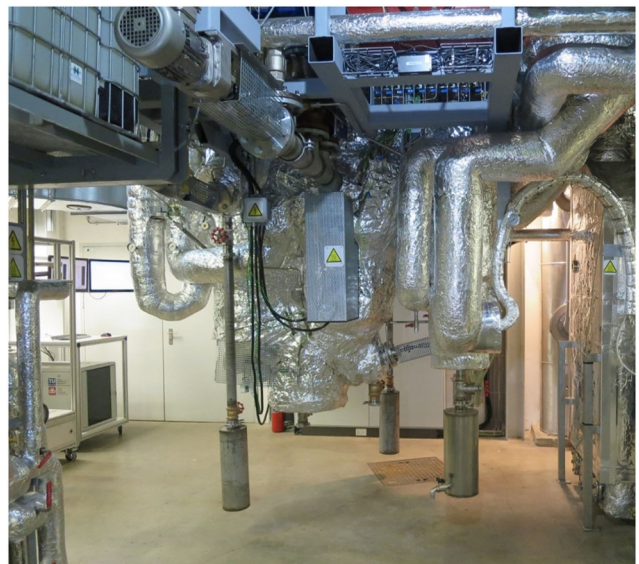
Fig. 4 Lower part of the 100 kW th gasification pilot plant, TU Wien [28]
