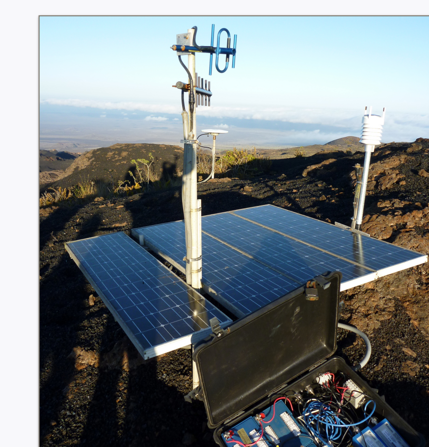
Figure 3 (above): A completed GPS site on the caldera rim of the Sierra Negra volcano, Galapagos Islands. The station includes an array of equipment types: GPS antenna and receiver, solar power source, batteries, radio transmitter, and meteorological equipment.
