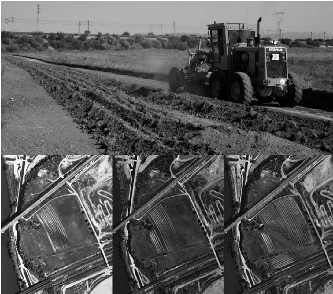
Fig. 5. Mechanical ground stripping performed by a motor grader and evolution of the stripped area in 2007, 2008 and 2009
