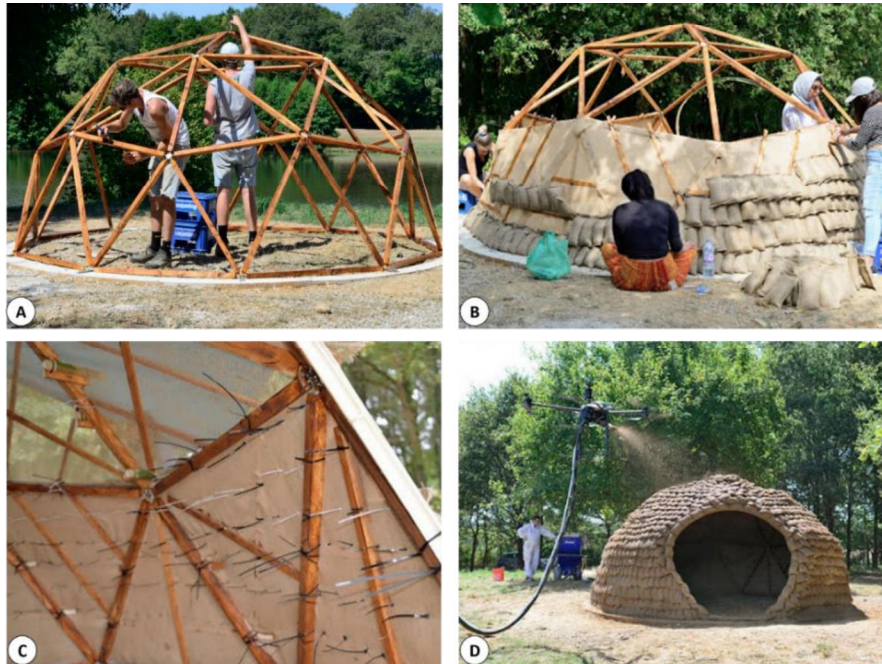
Figure 5: CS2: A) installation of wooden formwork, B) attachment of hay bags, C) formwork detail, D) drone spraying
