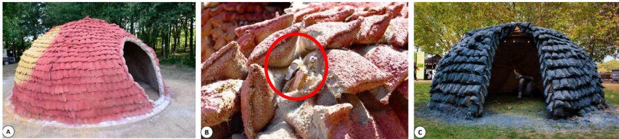
Figure 6: A) Finished dome sprayed with paint for waterproofness, B) Failure of prefabricated hub, C) London dome
